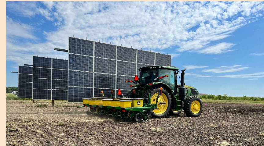
Installing solar panels in agrivoltaic systems Photo credits: SCAPES project (award no. 2020-68012-31934)
