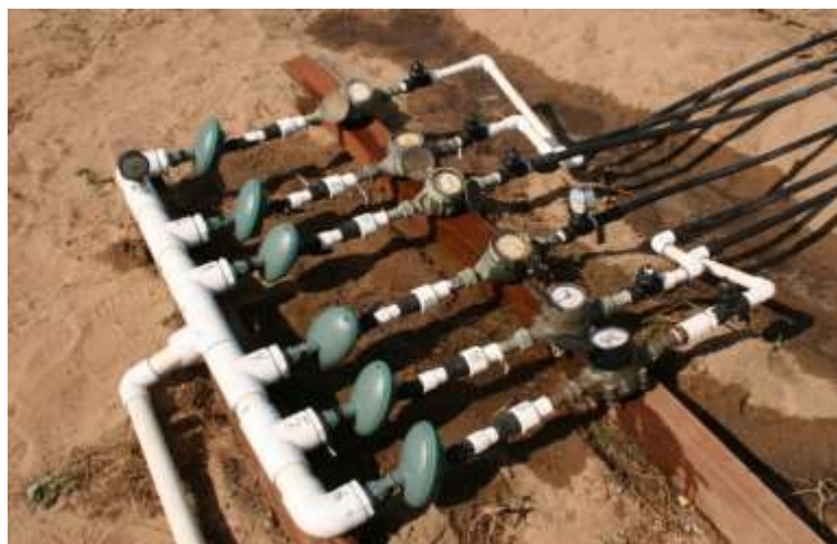
Figure 2. Irrigation control manifold.
