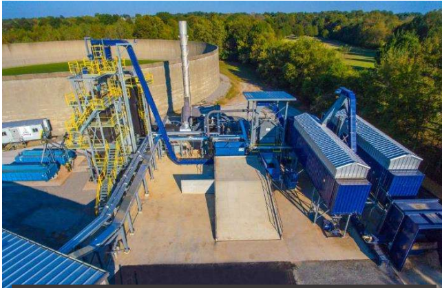
Downdraft gasification system in Lebanon, TN.
