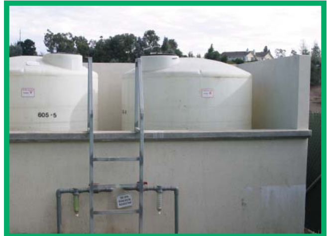
Example of secondary containment around fertilizer tanks.
