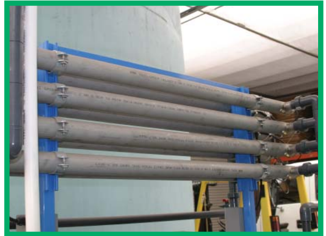
Example of an ultraviolet(UV) treatment system.
