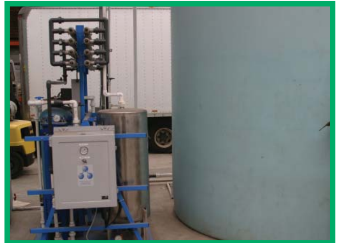
Example of an ozone treatment system.
